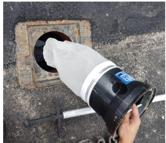
Photo 7: Containment strategy: Drains fitted with filter.
