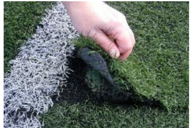
Photo 17: Example of seam becoming undone and can cause a trip hazard (source: Alastair Cox Associates)
