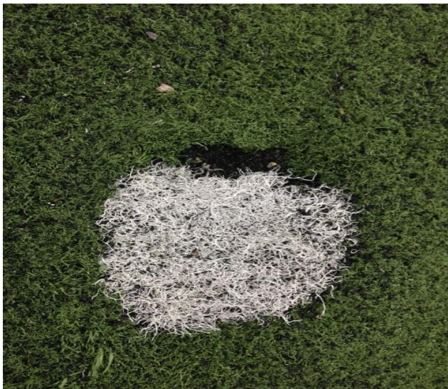
Photo 13: Heavy wear area of penalty spot that needs replacing as dangerous trip hazard (source: Smart Connection Consultancy)
