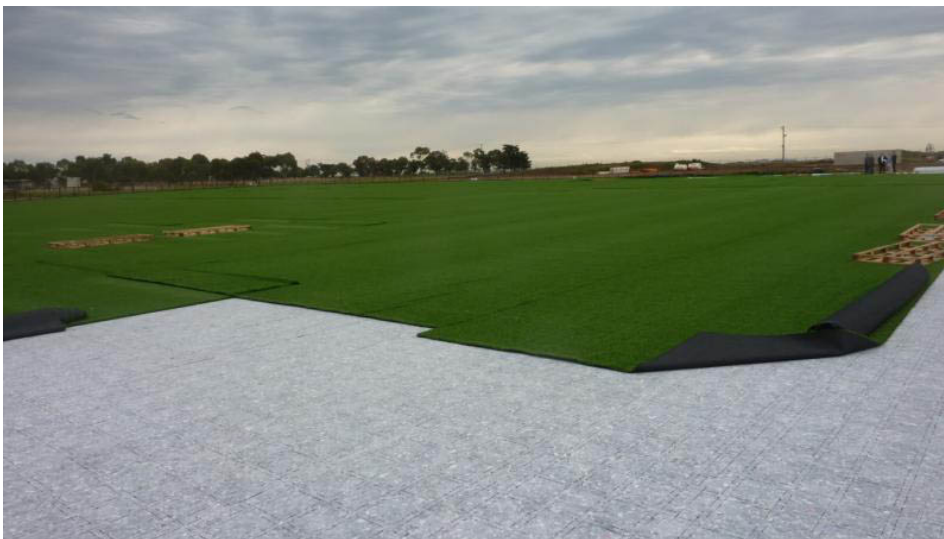
Figure 1: Construction of the first AFL and CA endorsed synthetic turf oval in Australia at Point Cooke, Melbourne.
