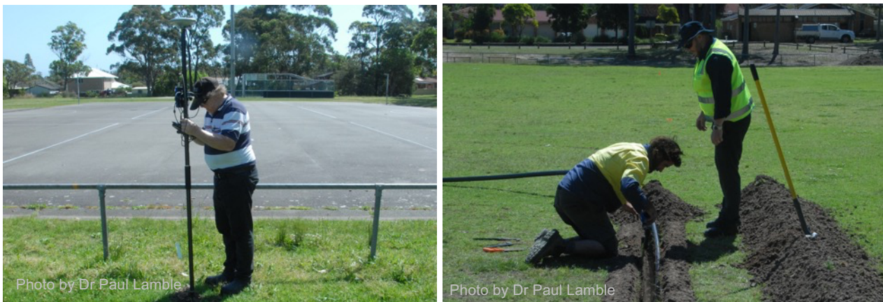
Figure 17.4: A certified irrigation designer completing the GPS survey of the irrigation installation (left) and a council officer inspecting sprinkler installation (right).
