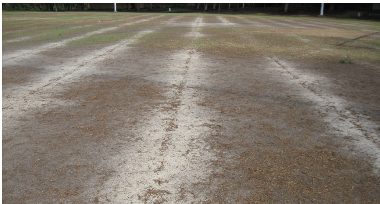
Figure 14.9: Slit drainage was installed in this field which needed the soil amended and the turf cultivar changed to handle the current usage levels. By performing these works in the wrong order, more funds will be needed to reinstate the slit drainage which will be buried during the soil and turf works.
