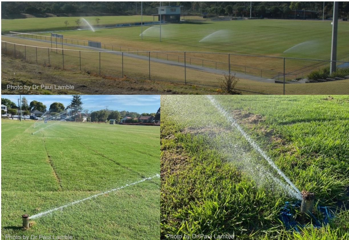
Figure 11.3a: Examples of poor installation practices including lack of coverage and sprinklers spaced too far apart (upper picture) and low operating pressure (lower pictures).
