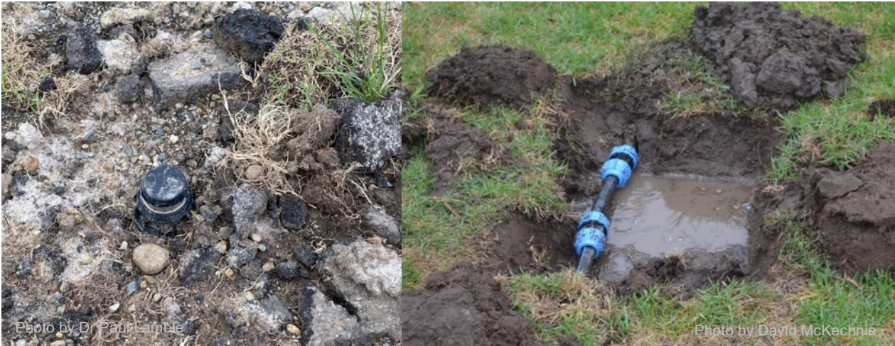
Figure 11.3b: Examples of poor installation practices including inappropriate material used as backfill around sprinklers and in trenches (left) and pipe installed at shallow depth preventing aeration (right)
