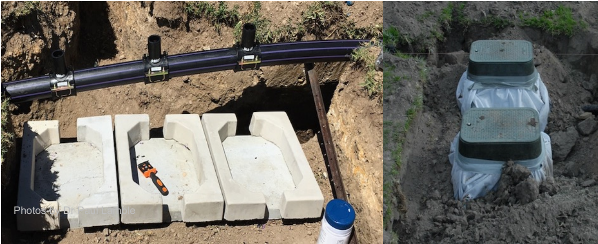
Figure 11.4: Irrigation installation examples. Electrofusion fittings for connection to the irrigation main line, paving slabs and c-sections for valve box supports (left) and valve boxes wrapped in geofabric (right)
