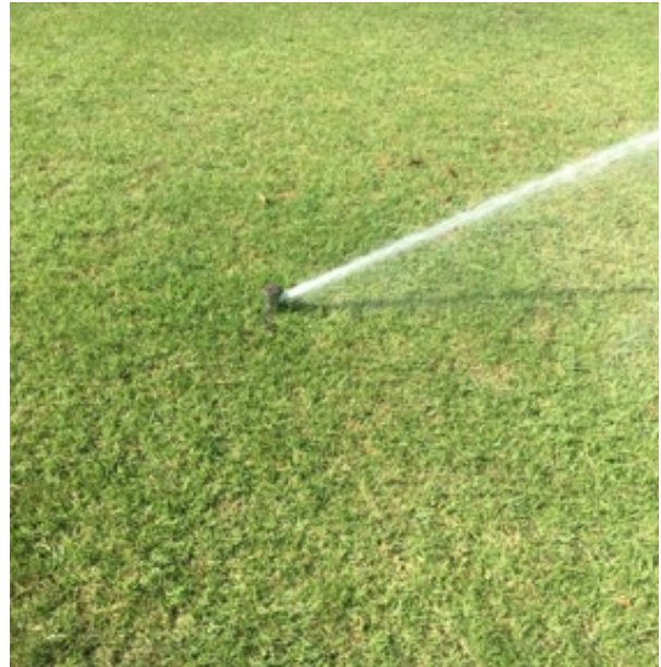
Correct sprinkler height
