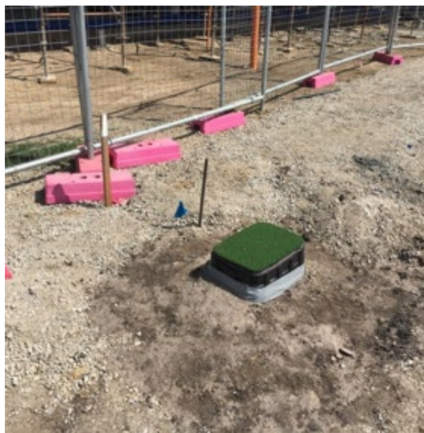
Installed solenoid box
